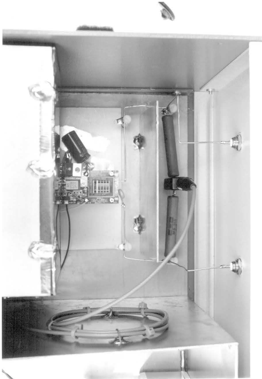
Figure C21 • Calibrator Section Detail. Inverter in Center with Load Resistors and Current Transformer and Current Transformer in Foreground. Note Shield Between Inverter and Load Resistors, and Low Capacitance Layout
